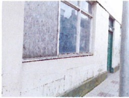
The Old Court House 53 Main St unoccupied more than 10 Years
